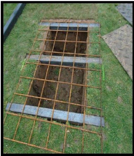
Tubular Supports and Grid
