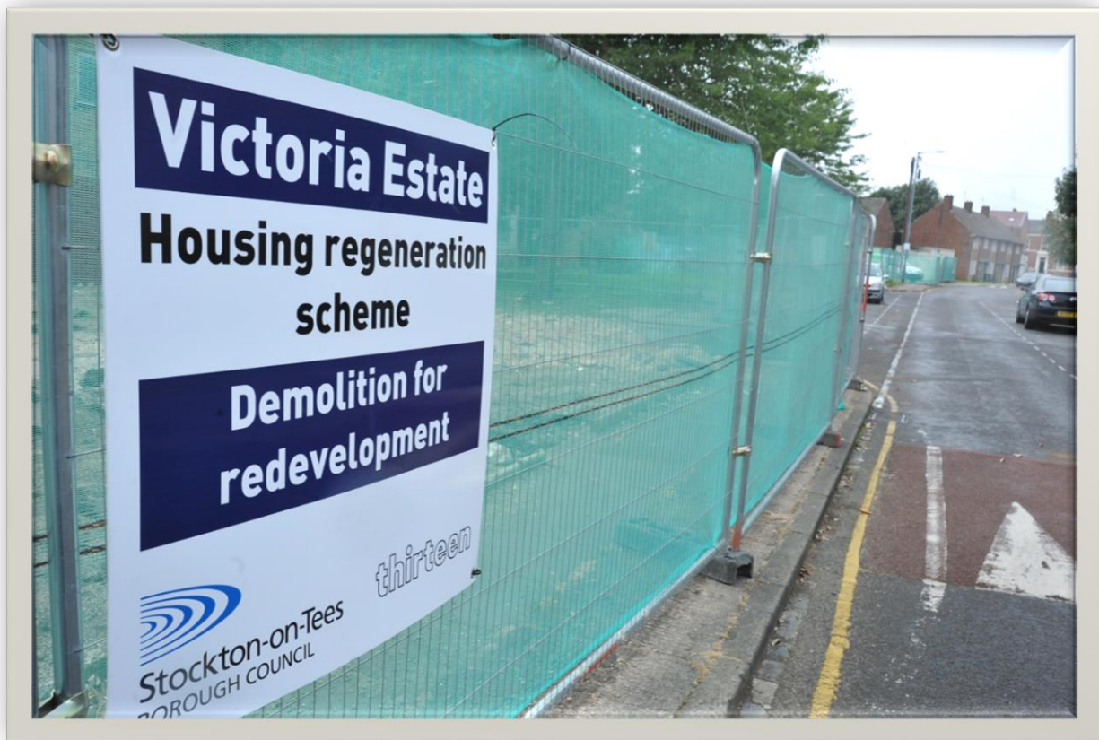
2016 saw the start of the Victoria Urban Village Living (promoting active and healthy ageing) development in Stockton Town Centre
