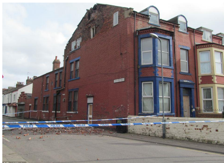
Collapsed gable end on Grove Street, Stockton after storm in March 2013
